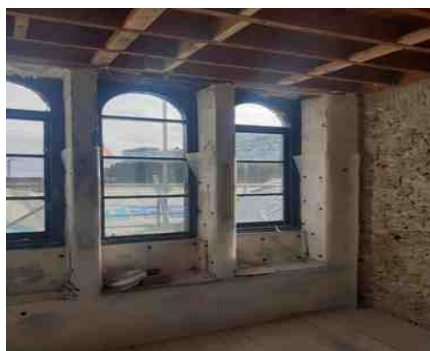
The First Floor of the Watchtower showing the delta membrane being installed.
