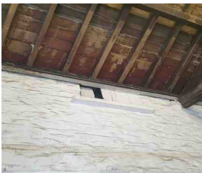
When stripped back you can see the windows that were originally part of the Custom House (now Pier Café) and then were obscured when the Lifeboat Station was built in 1866.
